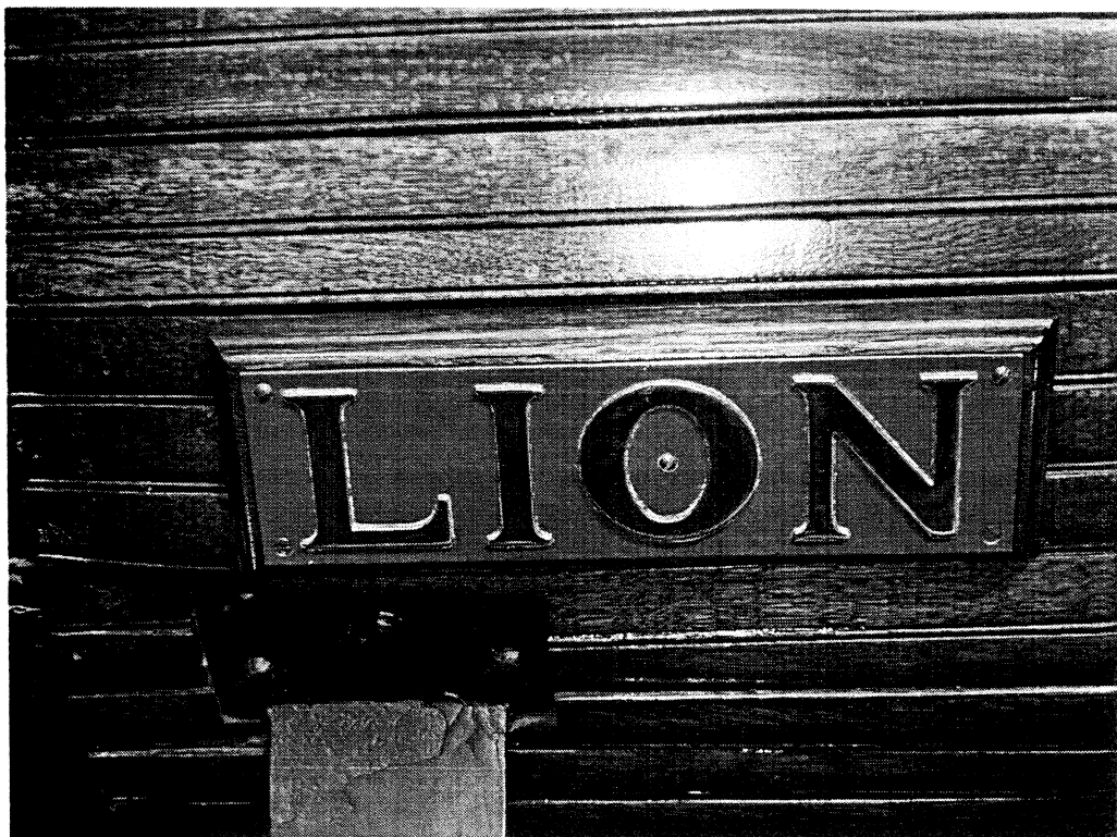
Detail of the boiler cladding and brass nameplate. Note the warping in the cladding to the left of the nameplate.
